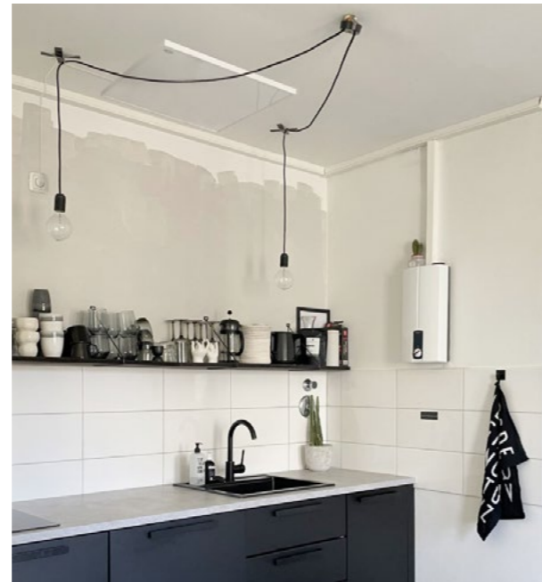
Ceiling heating in the kitchen.
